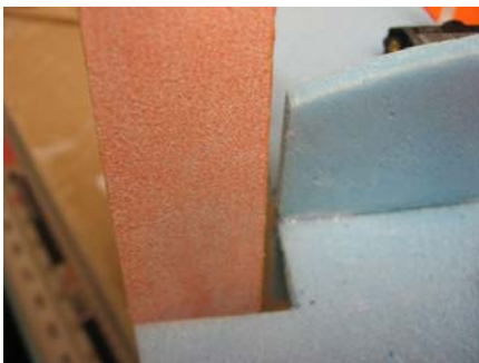
Photo #5 (sand area for repair)
